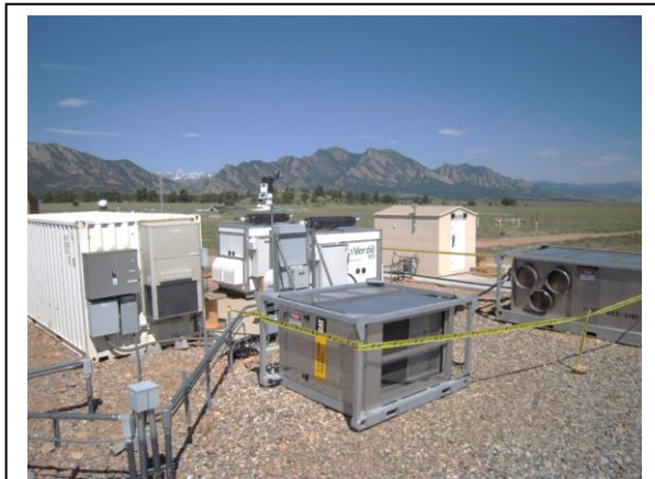
Microgrid equipment at the National Wind Technology Center in Colorado. | Photo courtesy of the National Renewable Energy Lab.
