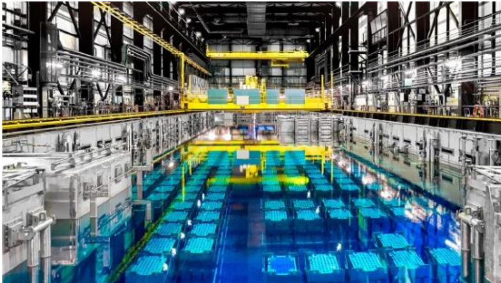
The Orano La Hague reprocessing facility. More than 34,000 metric tons of used fuel has been treated here since the site's operation in 1976. (Photo: Orano)
